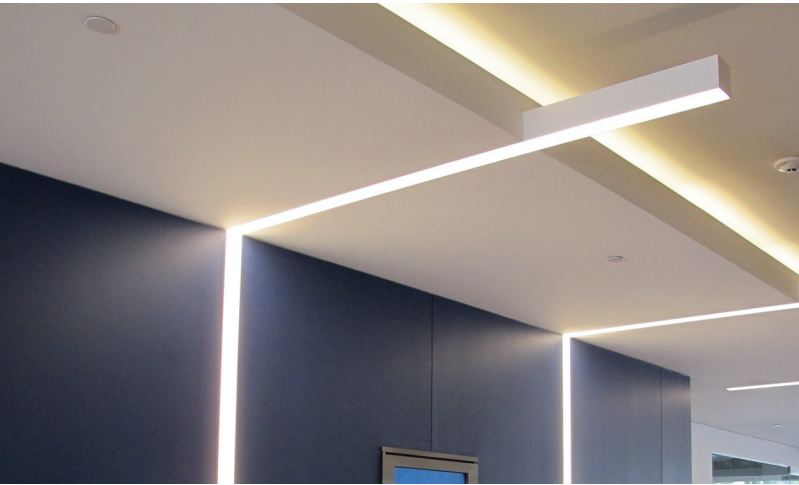
INTERIOR COVE LIGHTING
